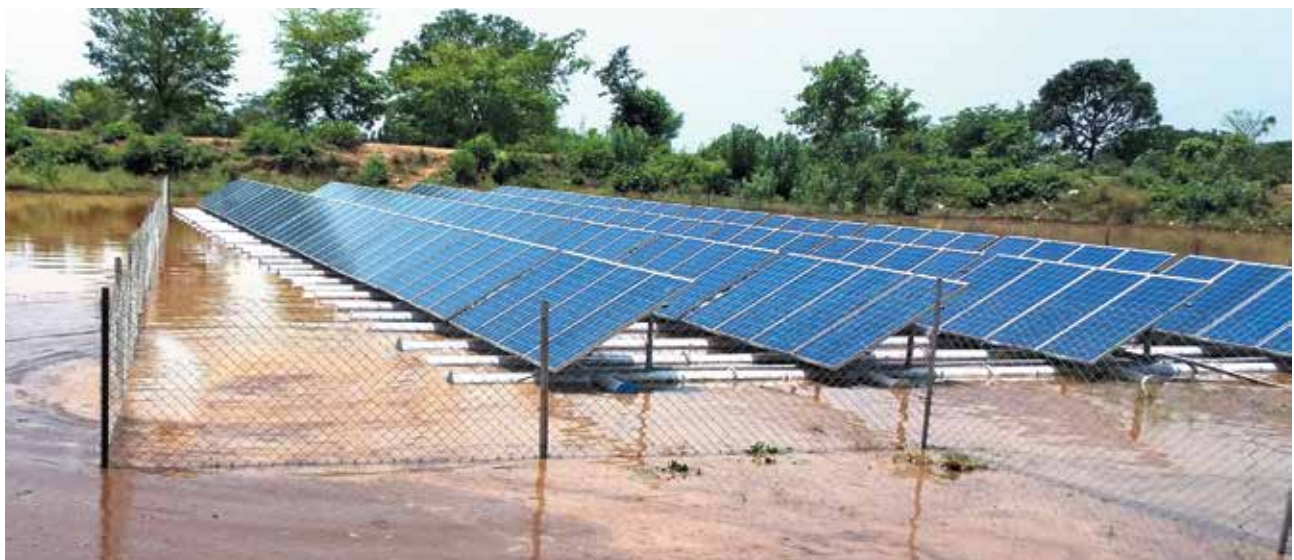
Jain Tarang (Floating) Platform in reservoir
