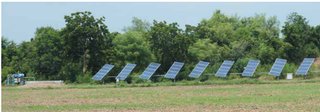
Solar Pump installed at Jain Tissue Culture Park, Jalgaon
