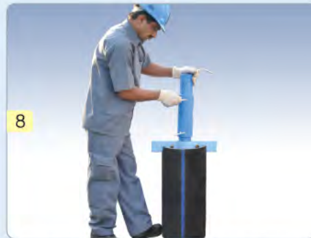
8 Repeat the Step 5,6 & 7 till all the pipes are lowered and connect the Top Connector
