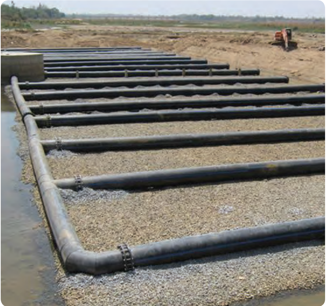
River Water Infiltration Gallery with Network of Slotted HDPE Pipes
